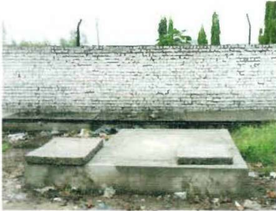
RWH -1 Location: Backyard Geolocation: 29.425941, 77.763470
