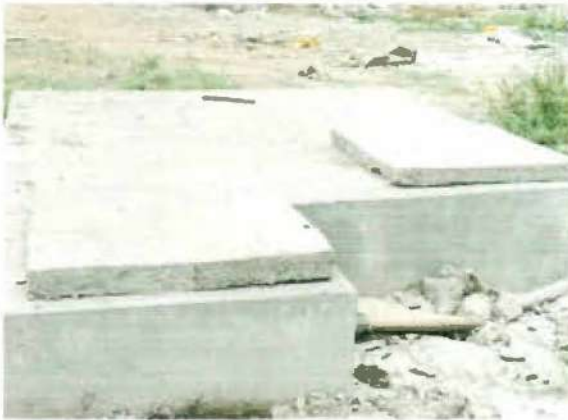
RWH -3 Location: Near pump house Geolocation: 29.427155, 77.762583
