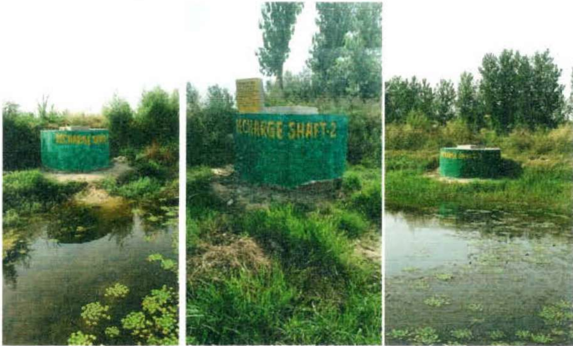
Fig 23: Photographs Showing Construction of 3 Recharge Shafts in Pond of Sikhera (Khasra No. 316/2)
