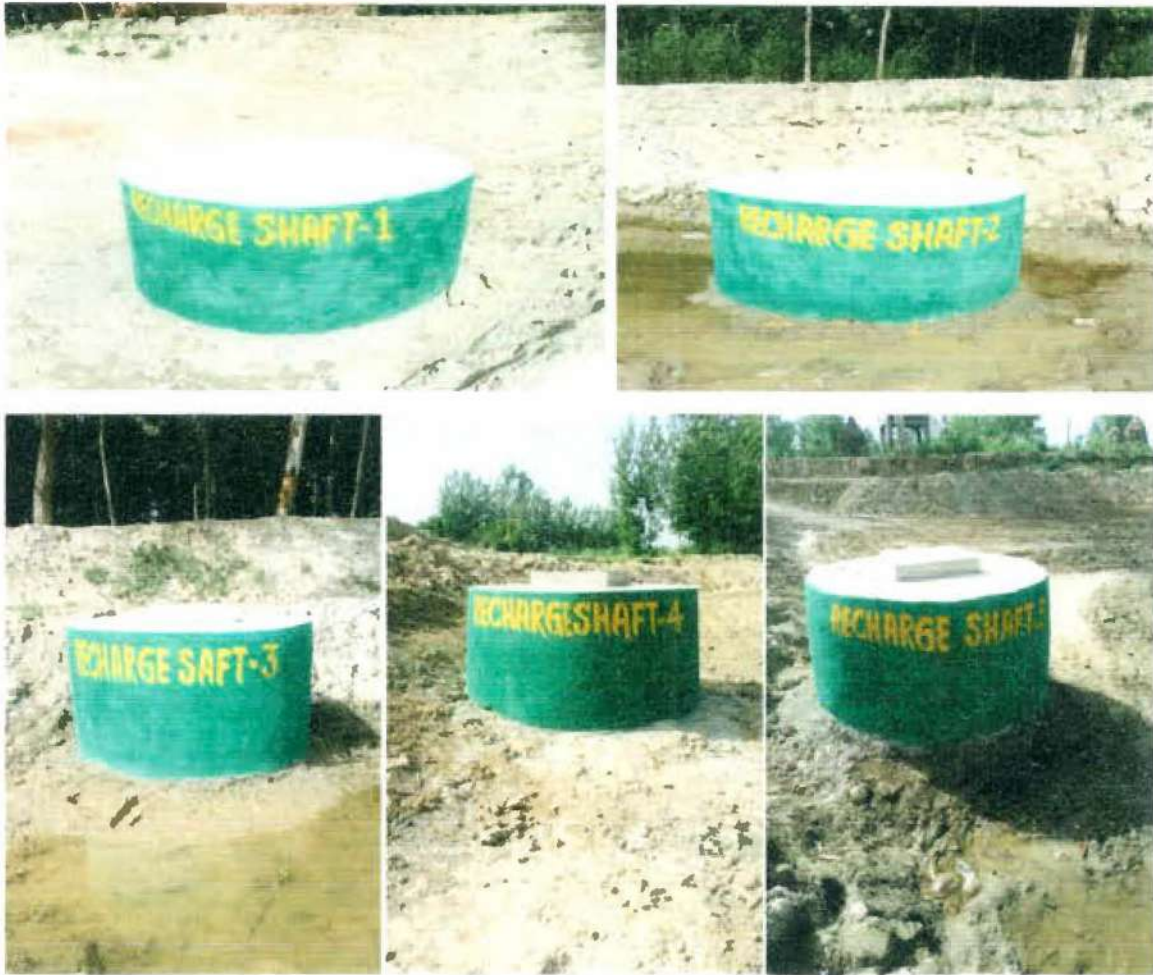
Fig 21: Photographs Showing Construction of 5 Recharge Shafts in Pond of Sikhera (Khasra No. 715)
