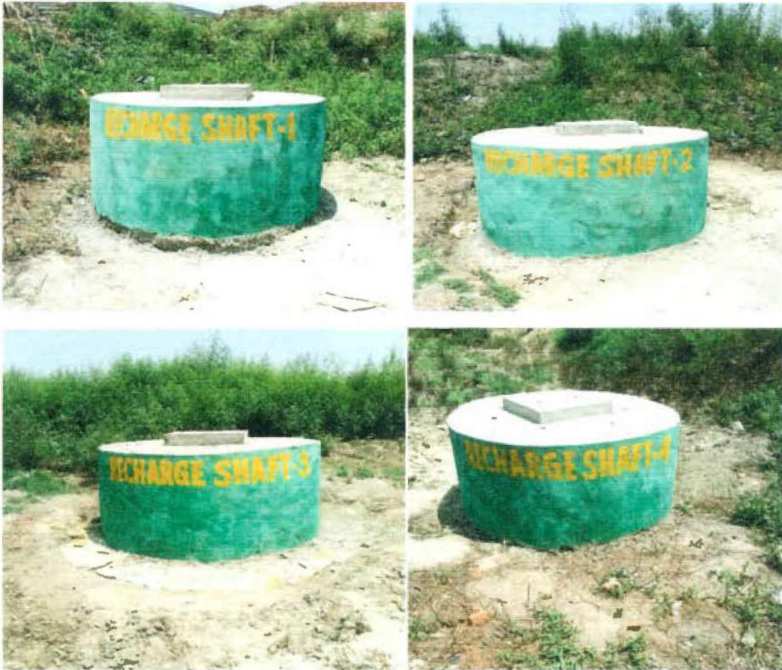
Fig 19: Photographs Showing Construction of 4 Recharge Shafts in Pond of Sikhera (Khasra No. 277)
