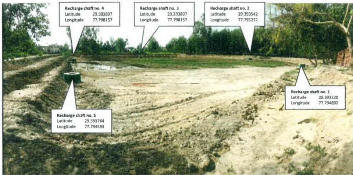
Fig 22: Photographs Showing Geo-Location of Recharge Shafts in Pond of Sikhera (Khasra No. 715)
